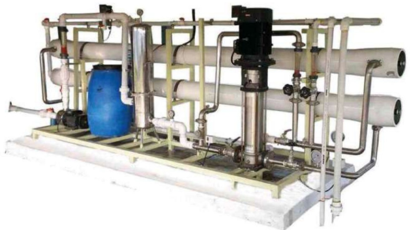
POST ETP - R.O. PLANT
